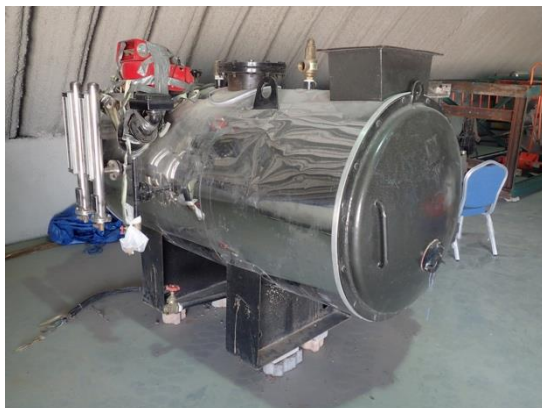
Figure D.36.7 Pressure vessel
