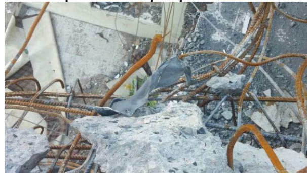
Figure D.60.5 Civilian apartment complex post blast
