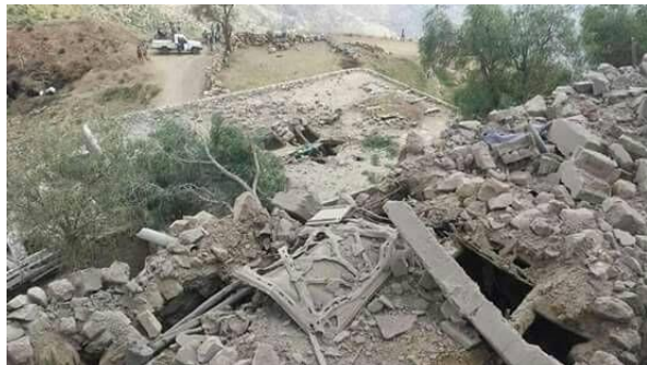
Figure C.58.4 Damage to al-Maqadhi houses (second strike)
